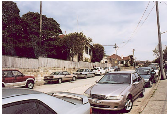
FIGURE 93 Sandstone block retaining wall with traditional timber paling fence above on the east side of Hopetoun Avenue
