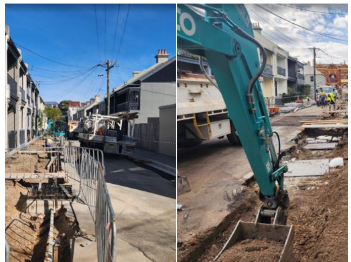
Sustainable upgrade of the stormwater system and streetscape in George Street, Paddington
