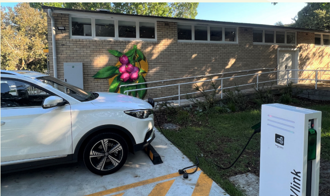
New EV charger at Cooper Park Community Hall.
