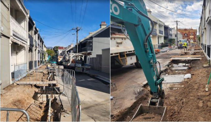
The Special Rate Variation supports us to achieve a significant uplift in tree and footpath investment, and the stormwater infrastructure that our community expects (pictured: sustainable upgrade of the stormwater system at George St, Paddington).
