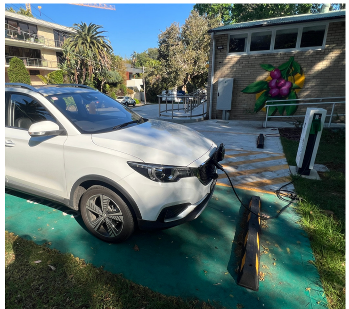
Electric Vehicle charger at Cooper Park Community Hall
