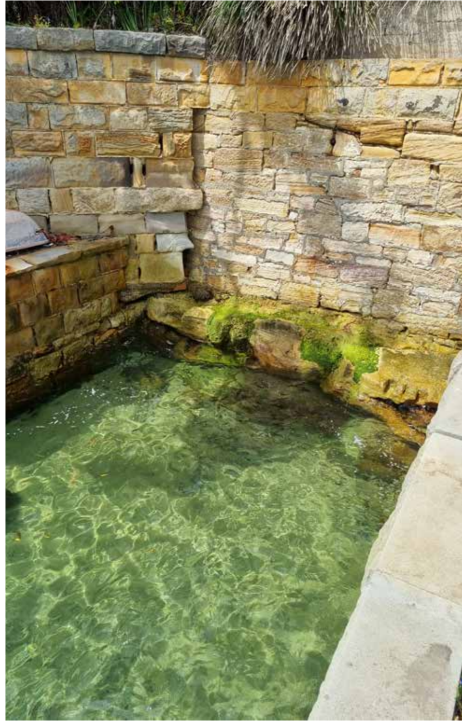
Remnants of Bath house foundations and lack of access to Darling Pt Reserve
