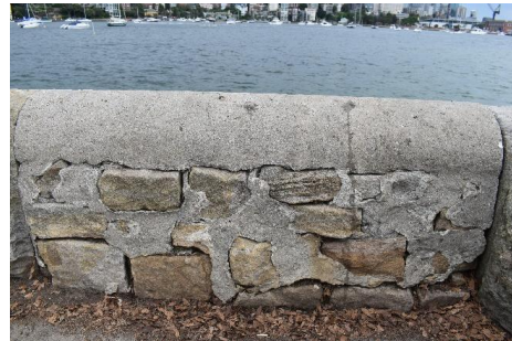
Figure 2.66 The stone repair to the seawall in the north of Yarranabbe Park. (Source: Ari Anderson, 2021)
